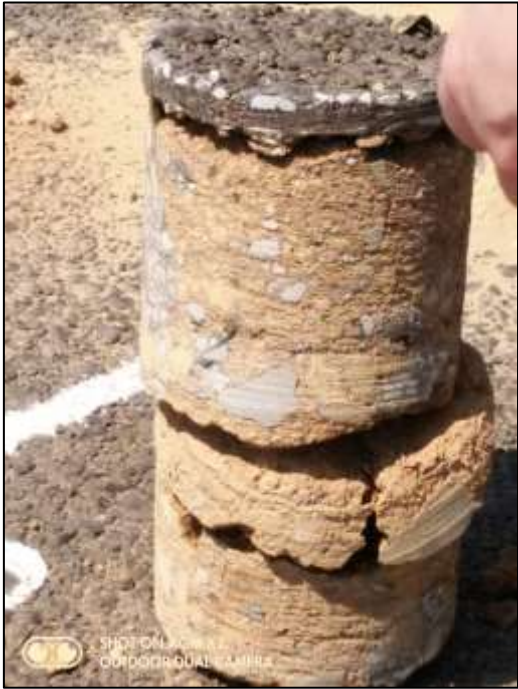
Photograph 2 (18 September 2018) Drilled core showing the double seal, 150 mm NME4 base-layer (1.5% NME) and 150 mm sub-base layer (1.0% NME) (NB: NO CEMENT !)
