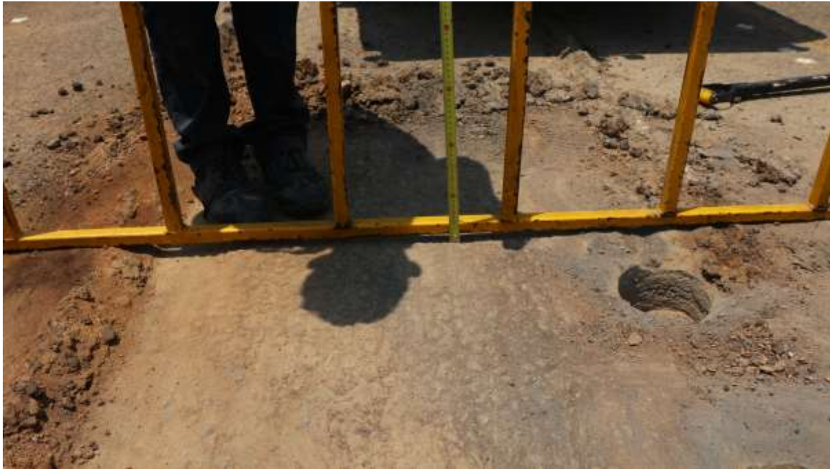
Photograph 6 (17 January 2019) HVS test site after removal of the HVS showing less than 10 mm rut depth
