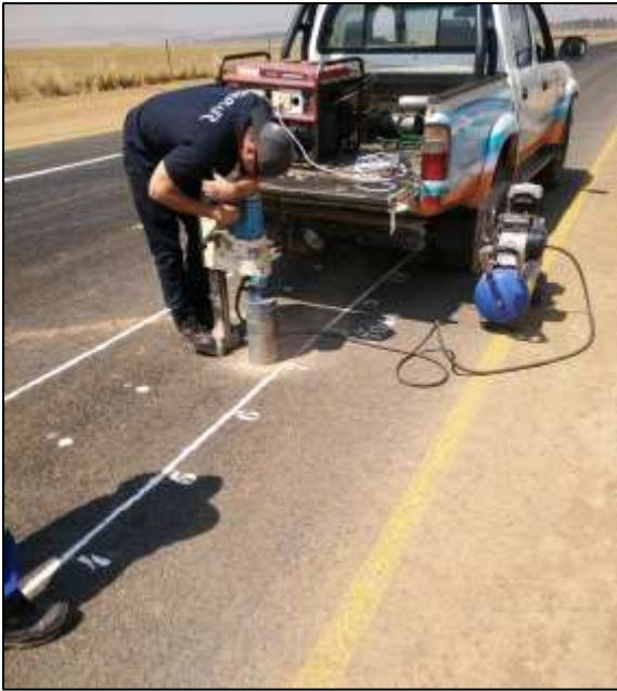
Photograph 1 (18 September 2018) Drilling of core on prepared HVS test site before start of HVS test
